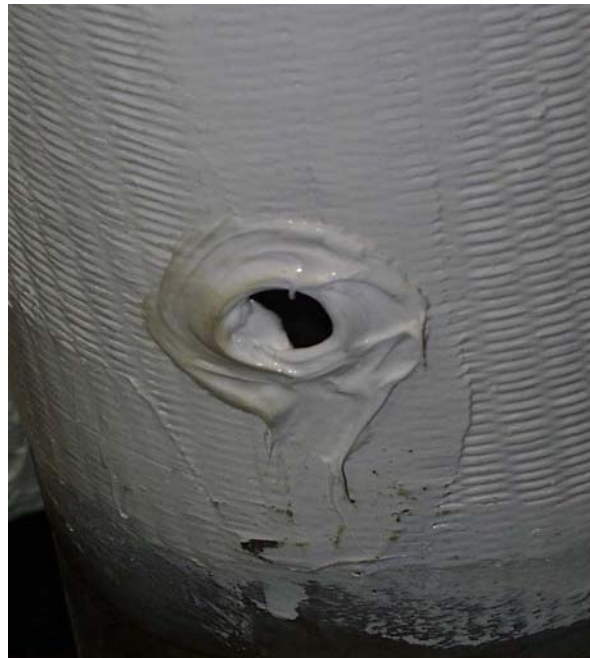
Figure 7.5 Access Hole on Wrapped Column
