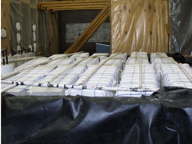
Figure 7.2 Irrigation Pipes Over Beams
